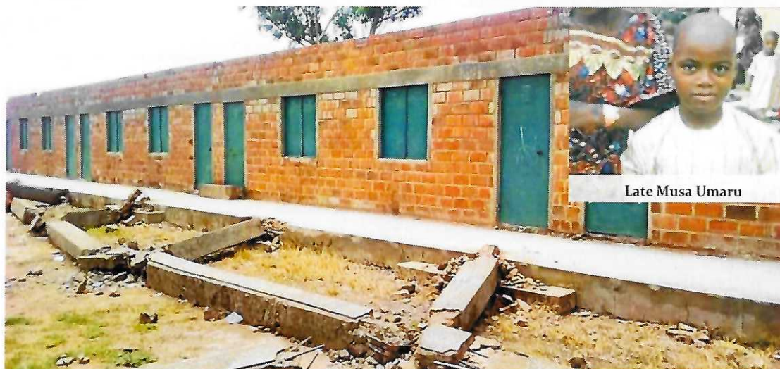
A poorly constructed school building which collapsed pillar tragically killed Master Musa Umaru, an 11-year-old pupil of Umar Isa LGEA Primary School, Dembo in Zaria Local Government Area of Kaduna State.
